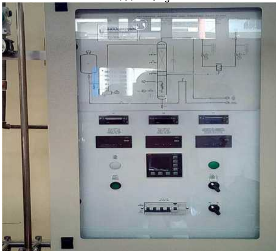
Panel de control
