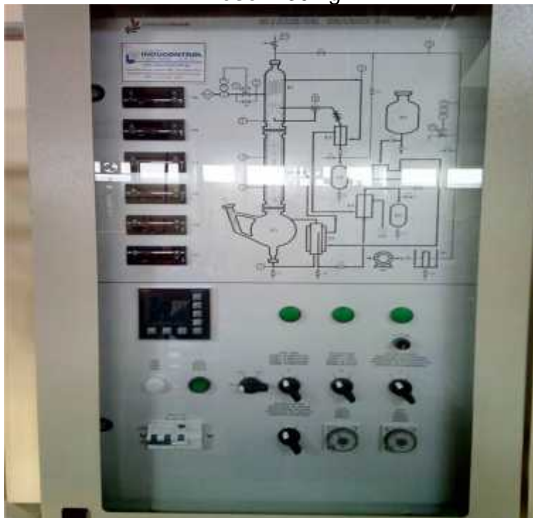
panel de control
